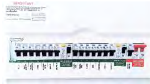
Utility Cupboard Consumer Unit
