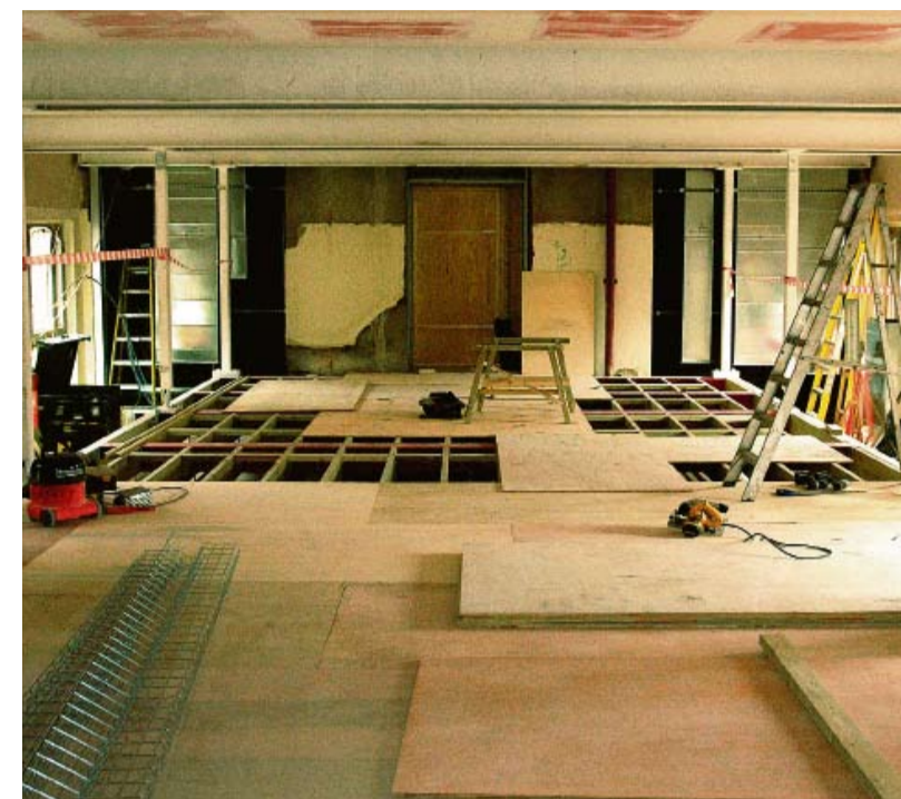
The mezzanine floor that will house the new and improved Student Activity Centre, with the Union Offices just below
