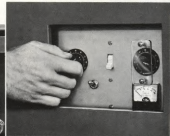
MAIN DRIVE AND TAKE-UP SPEED CONTROL PANEL
