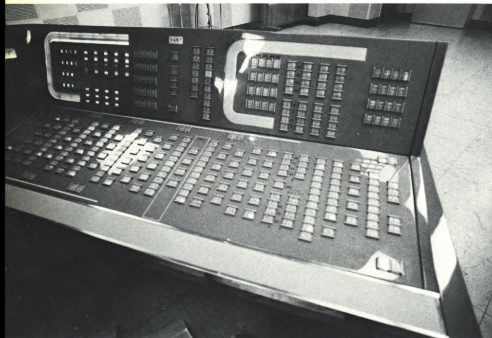
A section of the master control console showing push-button switches for establishing an almost infinite number of pre-sets. Pyrex red, blue and green filters on the cyclorama lights can, by percentage mixing, create all of the colors capable of reproduction by the television system.
